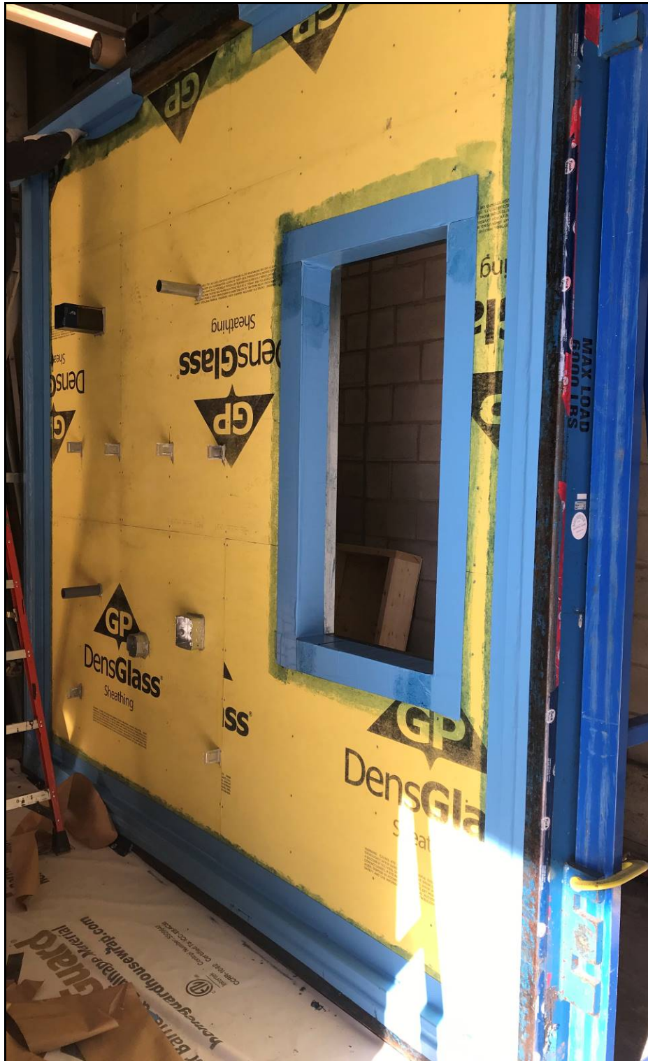
Photo H1 – Penetrations wall section; wall perimeter and window rough open prepared with membrane and penetrations sealed with sealant prior to product application
